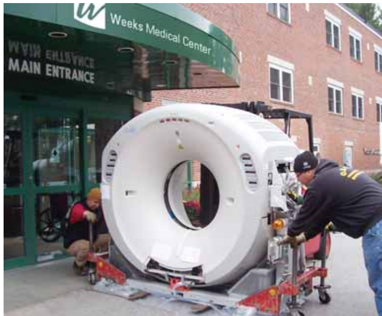
Installers moving the new 16 Slice Toshiba CT Scanner into its new home. This scanner replaced the single slice scanner.
